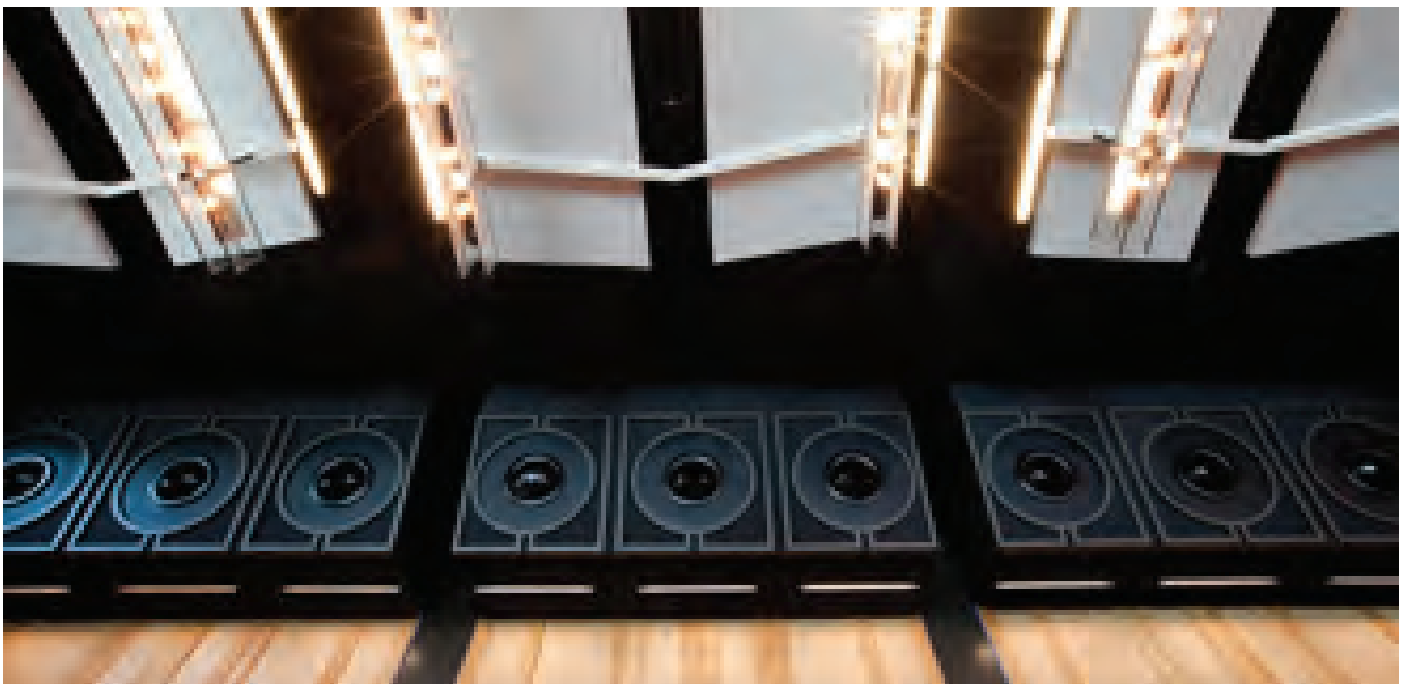
Figure 10 Air tight plenums containing three unique jet and perforated diffusers
