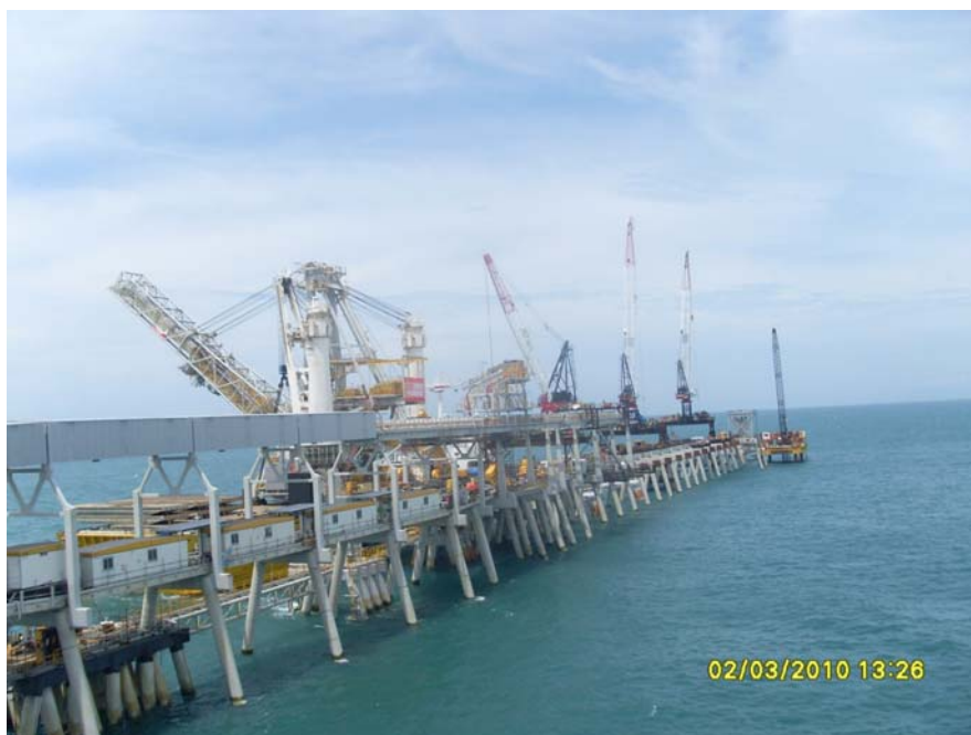
Figure 9 - Shiploader at APCT
