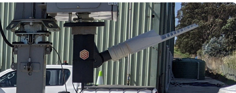
Above: The SiteHive environmental monitoring system had many benefits over traditional systems
