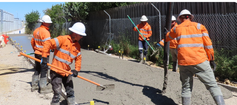
Above: Using eMesh, a recycled plastic material, to replace steel reinforced mesh – a Victorian first
